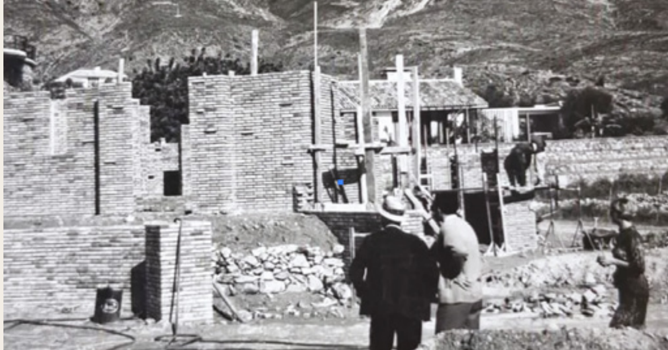
Robert Moshers observing the construction progress at Rancho Domingo in the 1970s.
