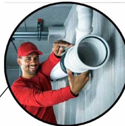
Tubes All plumbing tubes soundproofed
